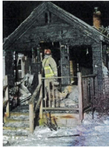
Fire-damaged house prior to demolition
