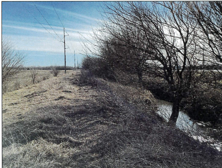
PHOTO 6: FROM THE NORTHERN POINT OF THE ACQUISITION FROM ON TOP OF THE BERM LOOKING SOUTHWARD AT THE BERM AND DITCH.
